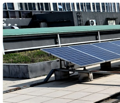
Photovoltaic Project of Wuxi R&D Center
