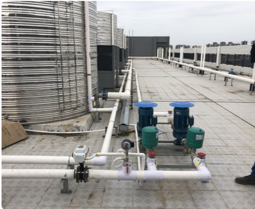
Pipelines for Waste Heat Recovery
