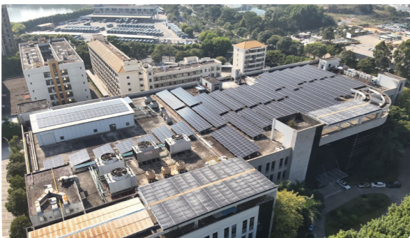
Phase I and Phase II Photovoltaic Projects of Dongguan No. 1 Manufacturing Center
