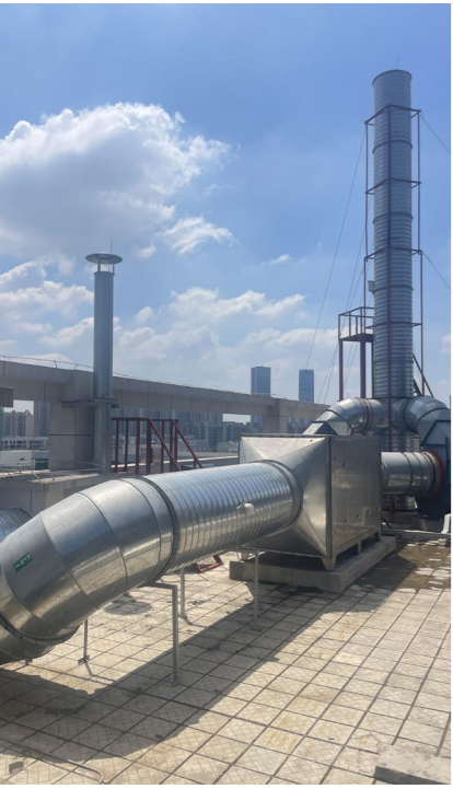
Activated Carbon Treatment Device
